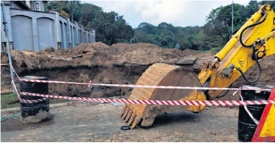
The excavation site had been left unfilled after work was carried out
