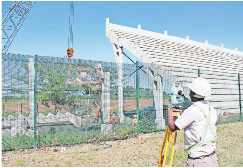
The construction team is working on the new open grandstand, which is steadily nearing completion Dave Savides
